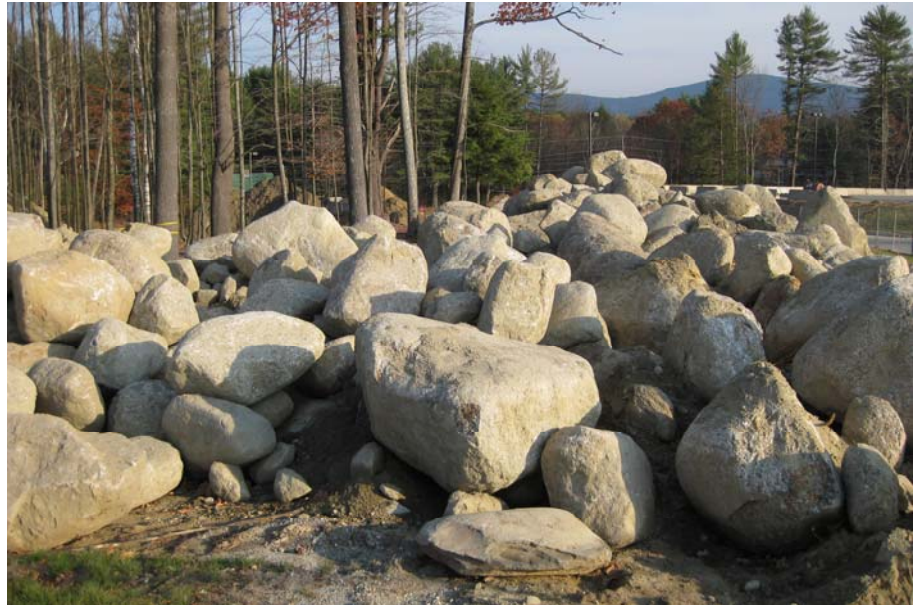
Rocks and small boulders that have been dug up during parking lot construction are being stockpiled. They will be used to create natural retaining walls in place of concrete.
